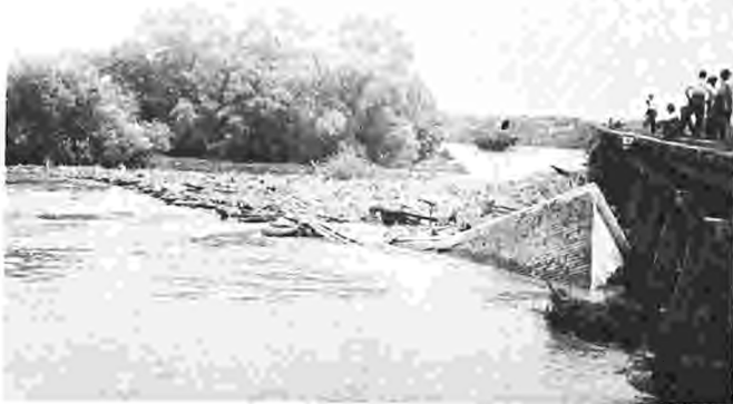
Debris at the Trestle
